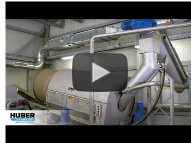
Video: HUBER Grit Treatment System RoSF 5 - grit recycling at WWTP Schwarzenberg
