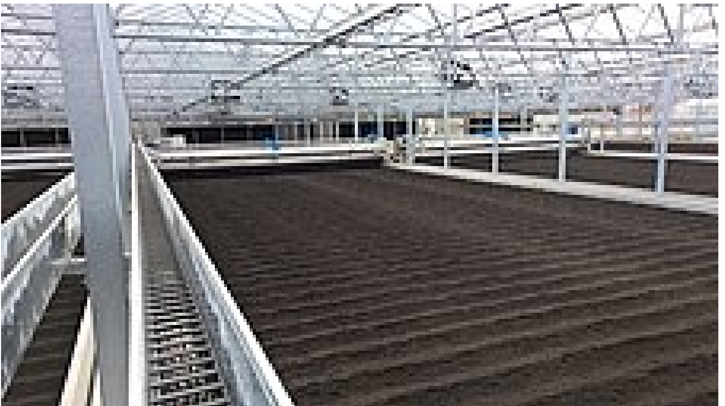
The sludge turner in the one-way road: The dry granulate is returned to the machine building
