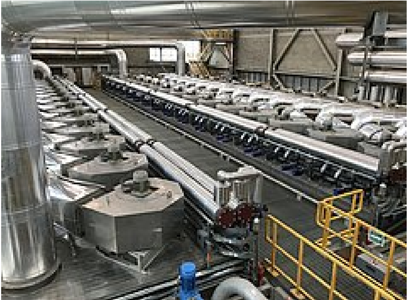
Impressive size: Three HUBER Belt Dryers BT 30 at new Bello wastewater treatment plant
