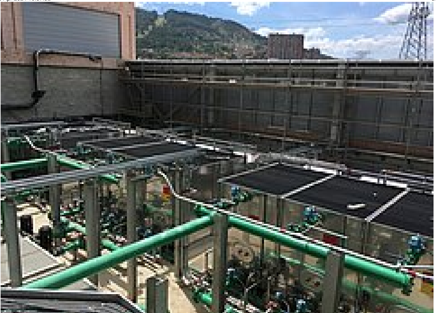
Cooling towers and exhaust air treatment
