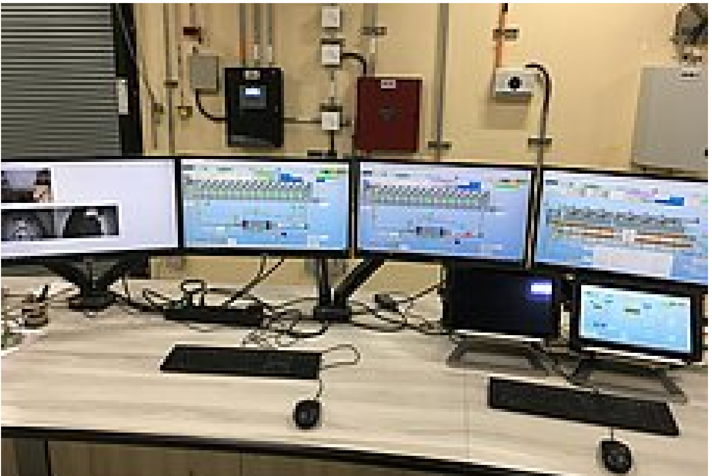
Control system for the drying plant
