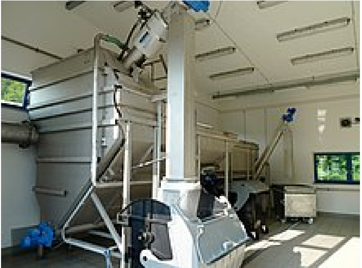
The plant in Ortenburg
