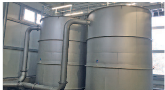
HUBER Active Carbon Filter CONTIFLOW® GAK as 4th treatment stage on STP Fridingen
