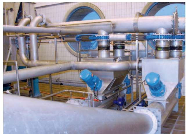
HUBER Launder Channel system feeding redundant HUBER Wash Press WAP® SL units
