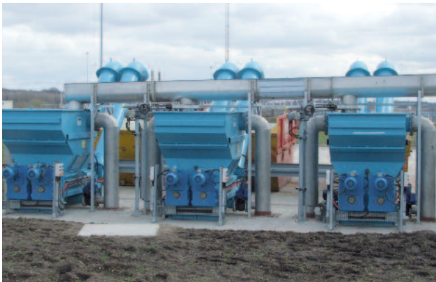
WWTP Knostrop (UK): 2 million PE HUBER Launder Channel HLC: 20 m 3 wastewater per second
