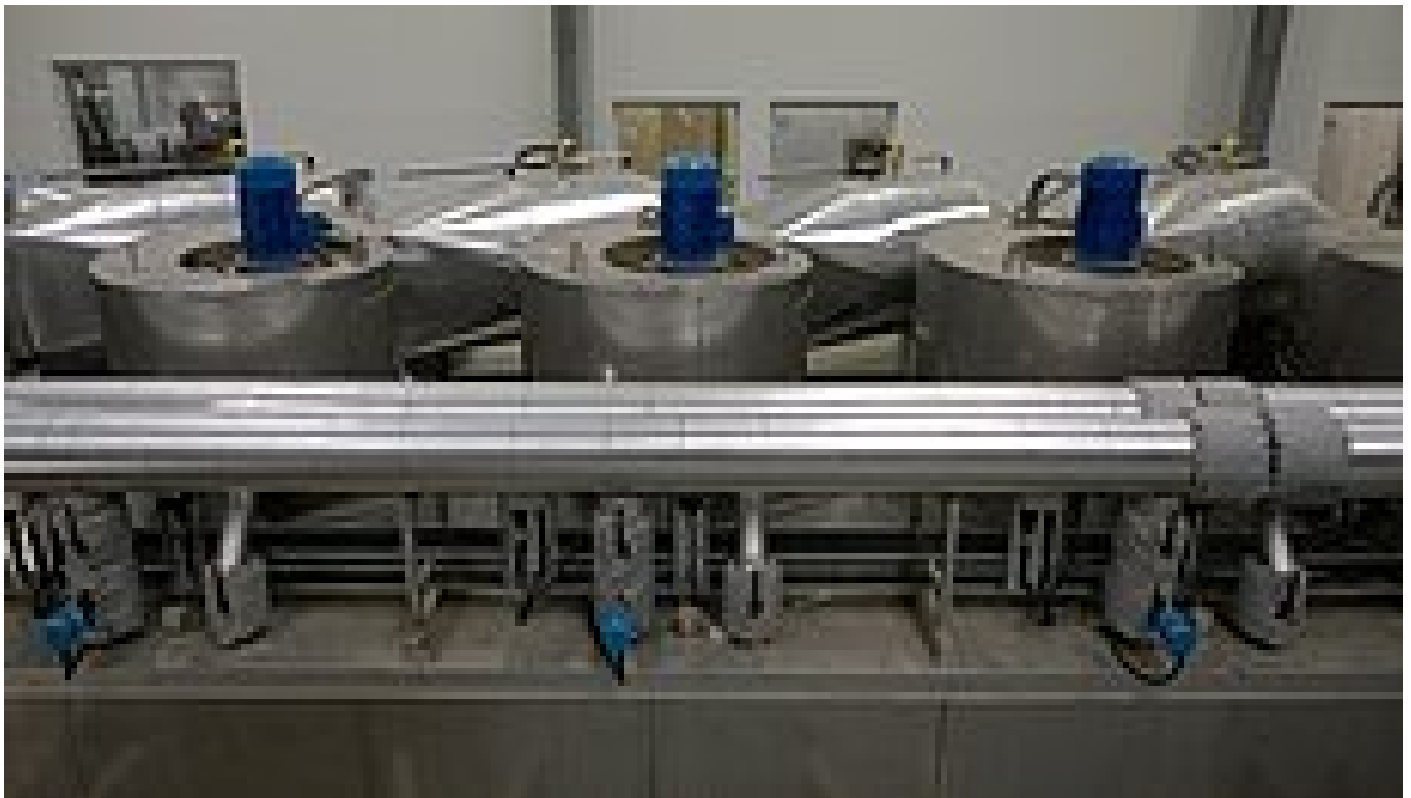
Hot water supply and ventilators of the sludge dryer with V4A insulation
