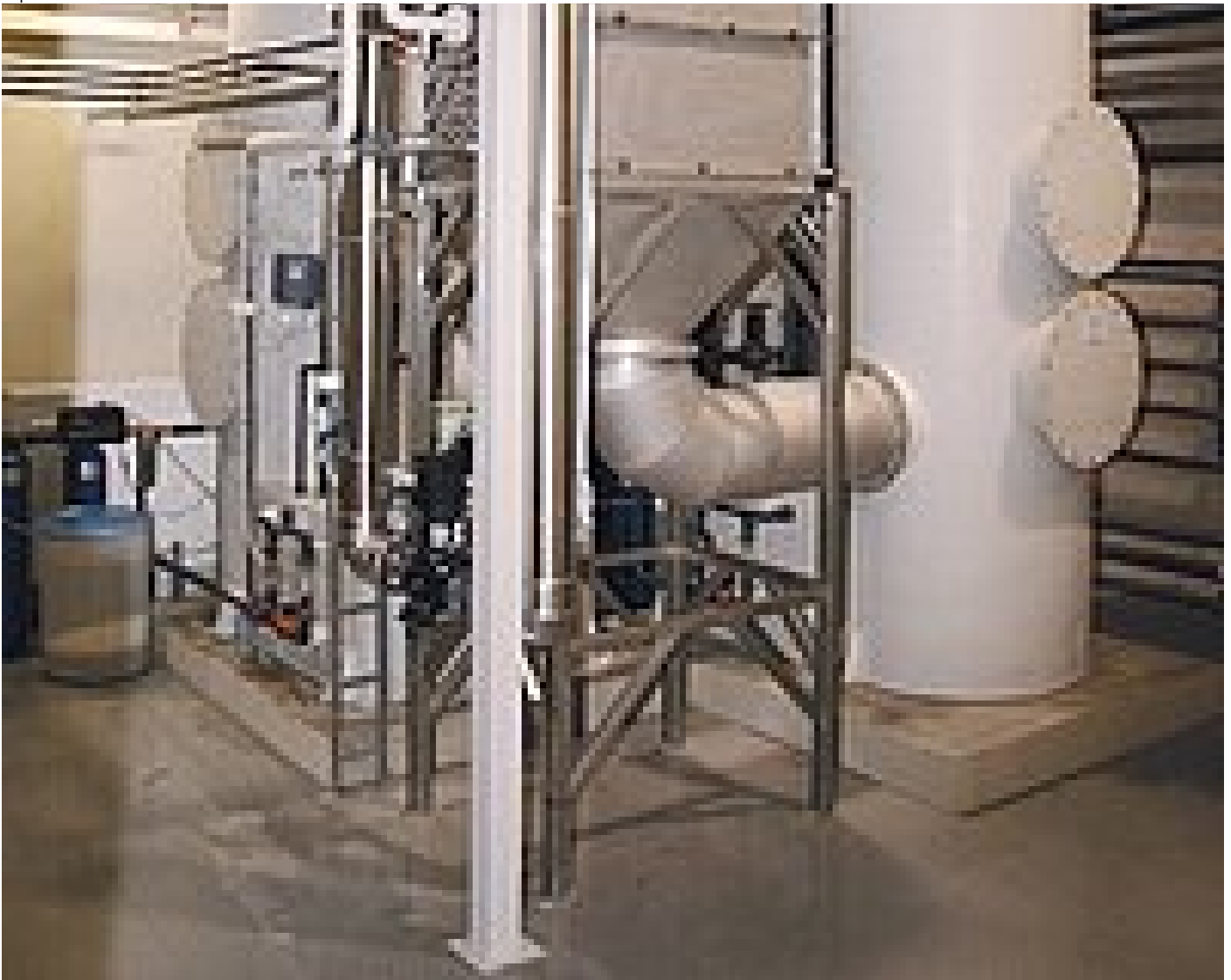
Heat recovery of the dryer and exhaust air treatment
