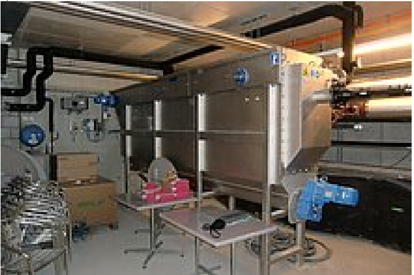
Figure 4: HUBER Heat Exchanger in the storage room beside the boiler room in the basement of the building
