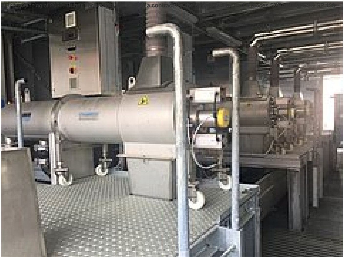
Series of STRAINPRESS® Sludge Screens installed at the East Rome WWTP.
