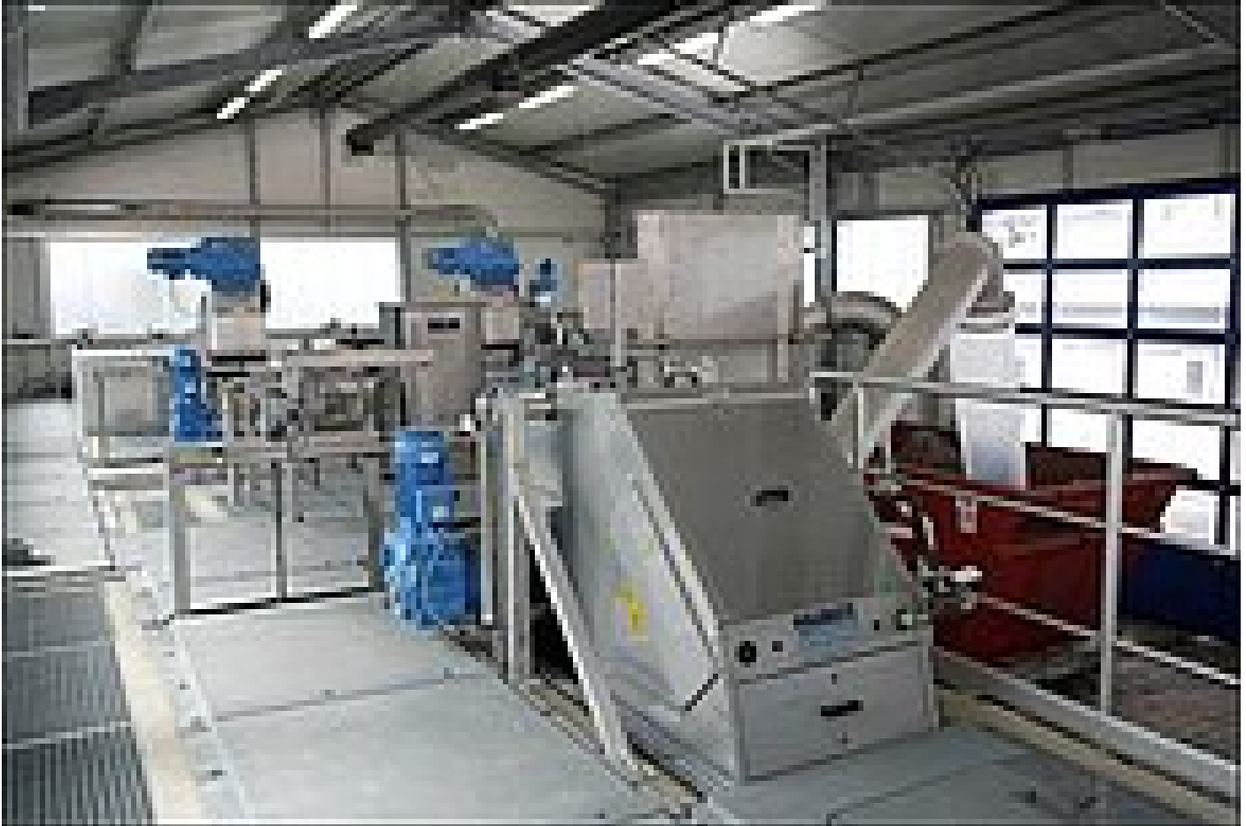
Coarse and ultra-fine screening at the plant in Glessen / Germany
