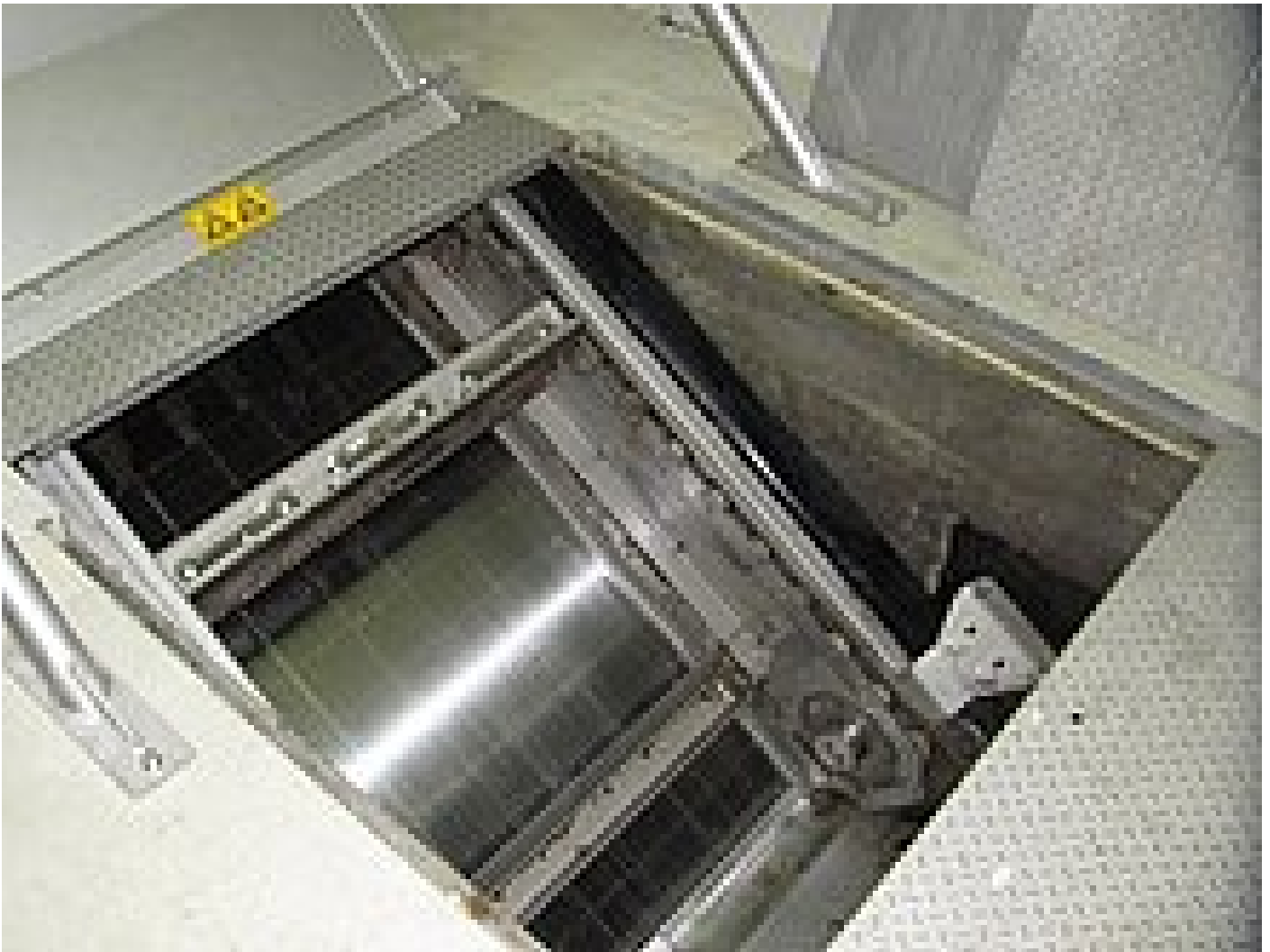
Due to the extremely flat installation of the bar rack the screen section through which the flow passes is always double the water level in the channel.
