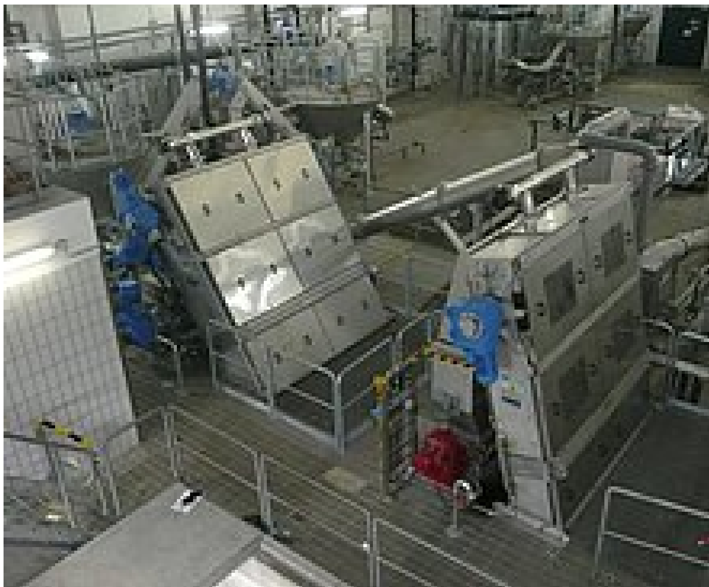
Line 1 shortly after start-up
