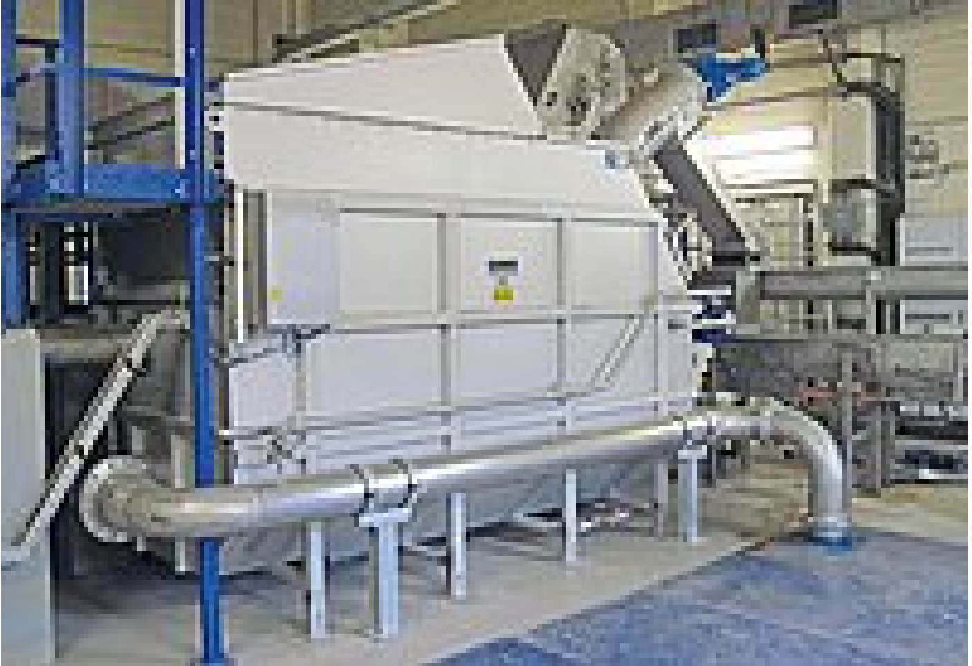
HUBER ROTAMAT® Membrane Screen RoMem Pro 1600 installed on STP Bitterfeld-Wolfen
